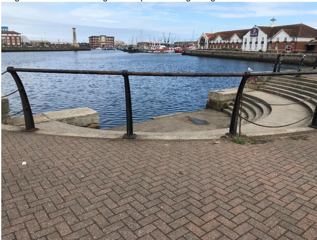
Image 2: Area demonstrating an example of missing railings and rust
