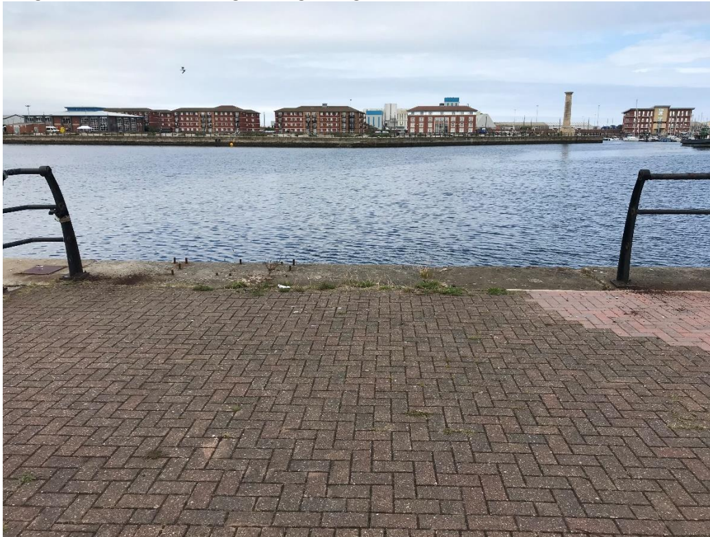
Image 1: Area demonstrating missing railings.
